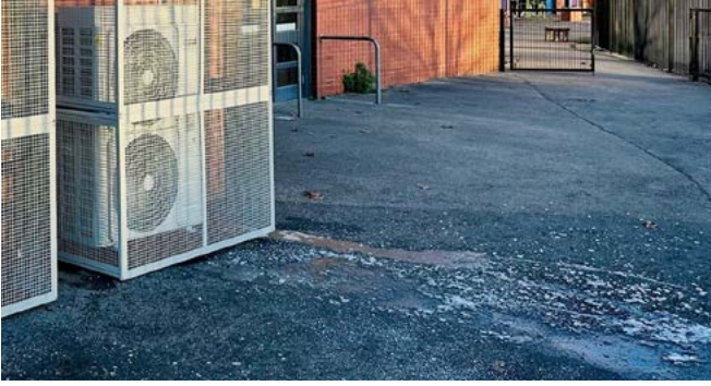
Condensate management should be considered for all installations.
