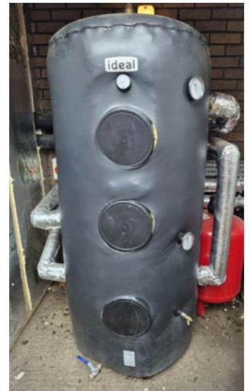
Ensure buffer tanks and pipework are sufficiently insulated
