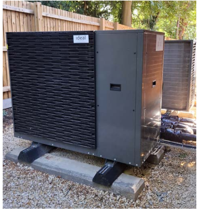
Two correctly sited ECOMOD 290HT 27kW commercial heat pumps in cascade.
